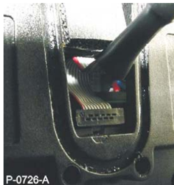
Figure 39: Excess Wiring Loom Cable Folded Correctly
